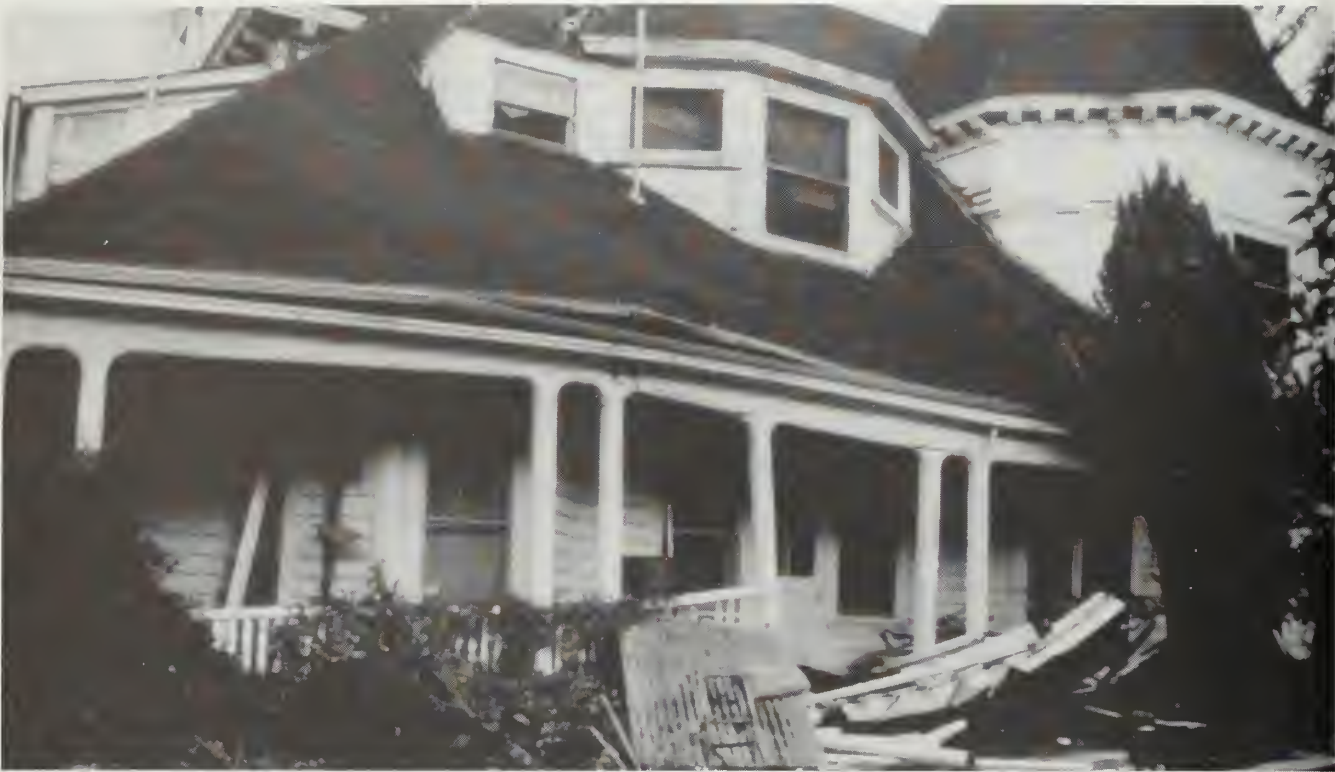
Collapse of a residence in Los Gatos during the 1989 Loma Prieta earthquake. The "cripple walls" of this old wood-frame house were unable to withstand the level of ground shaking experienced at 14 miles from the epicenter. Recognition of potential seismic hazards and appropriate retrofitting could have greatly reduced losses. Photo from Earthquake Engineering Research Institute.
